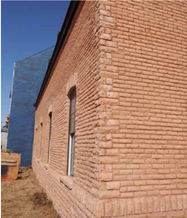
(Above) A close up view of the rock-face brick with its beautiful corner detail.
