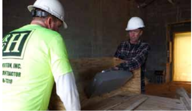
(Above) Workers examine a soffit model which will beautifully conceal ducting in the chapel.
