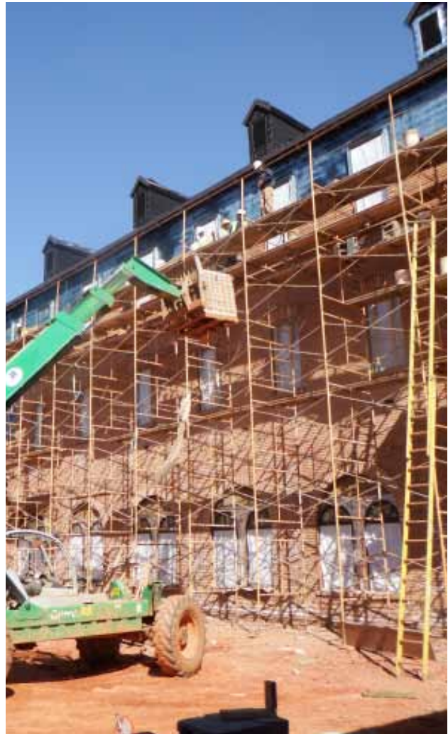
(Above) Scaffolding is rising up as the facade of the academic cloister nears completion.
