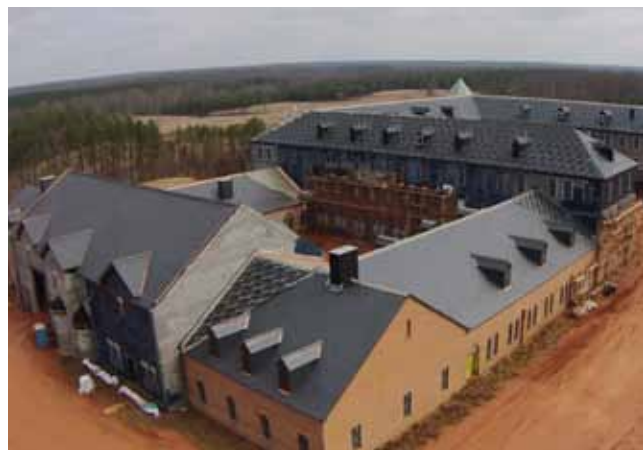
(Above) Slate and brick now cover large portions of the building's west face and roof.
